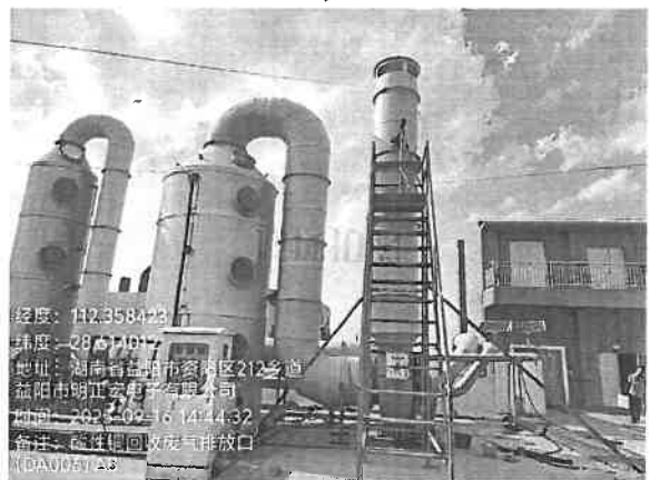
A 8 酸性铜回收废气排放口 (DA006) (E: 112.358423; N: 28.614012)
